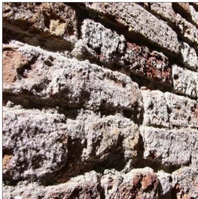
Figure 4 Salt crystals growth on brick surfaces [17].
